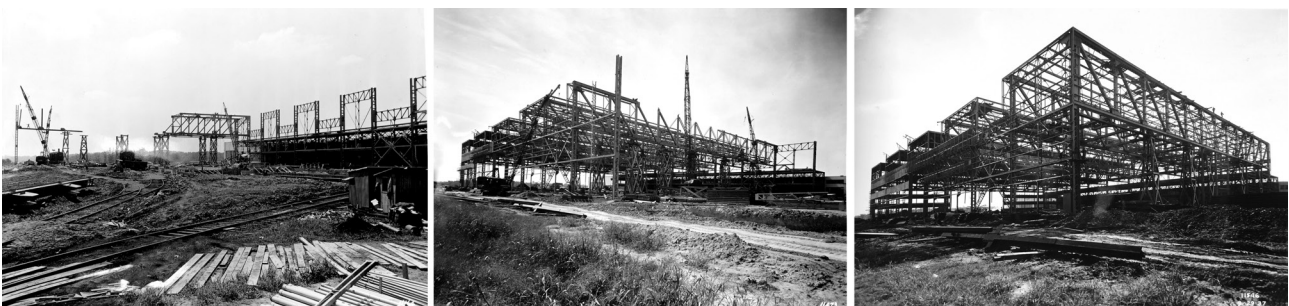
02. Albert Kahn. First extension of the Glenn L. Martin Co. Assembly Building. 1937. Consecutive photos of the development of the works.
